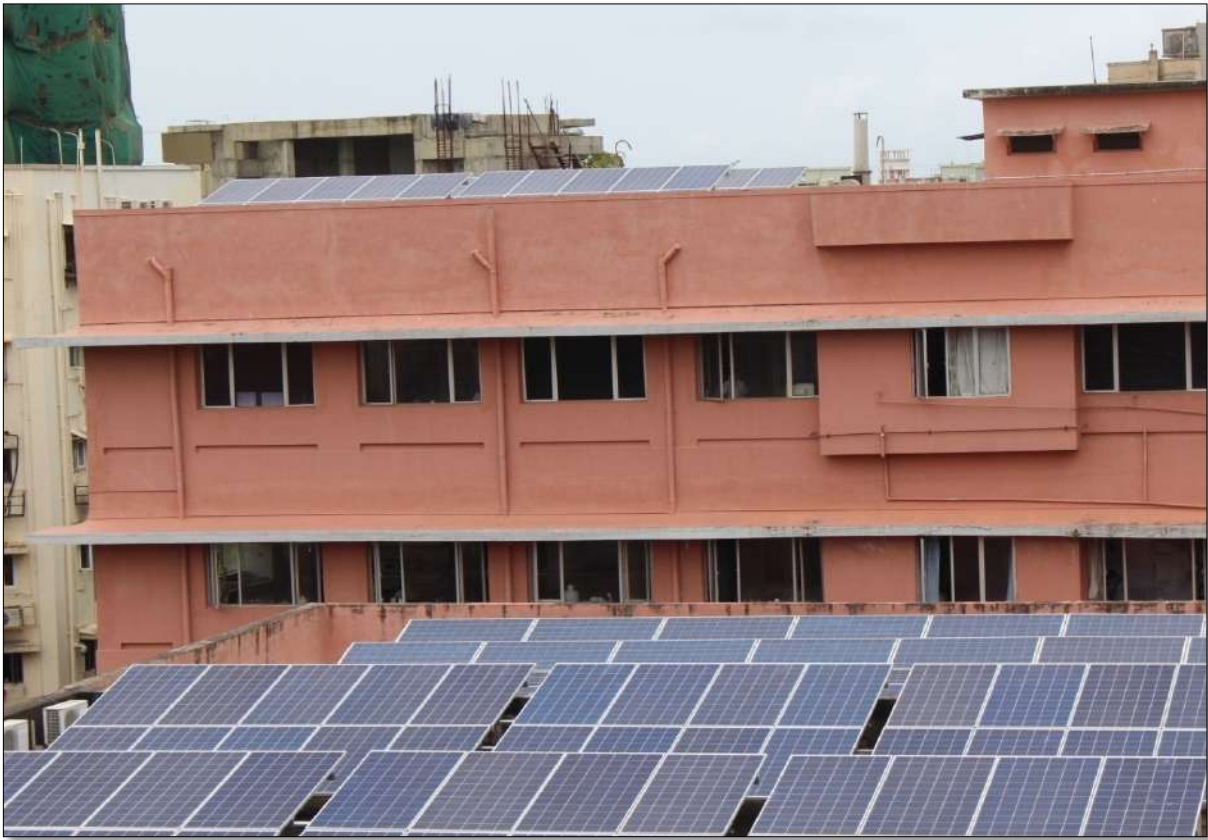
Solar panels – Main building
